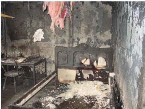
Damage to a bedroom from a candle fire
