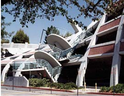
Earthquake – CSU Northridge (Jan. 1994)
