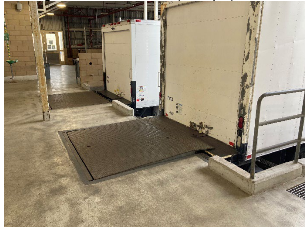
Loading Dock Leveler in Use (example)
